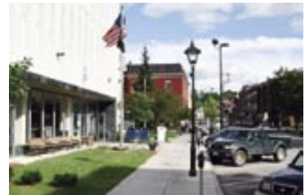
Sidewalks and streets outside the U.S. Post Office, Montpelier, VT were renovated in tandem with the city's reconstruction of a nearby water main.
